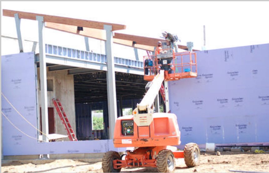
Construction continues on the Beloit Health System Cancer Treatment Center near the corner of Milwaukee Road and Lee Lane. Construction is expected to continue to the end of the year.
