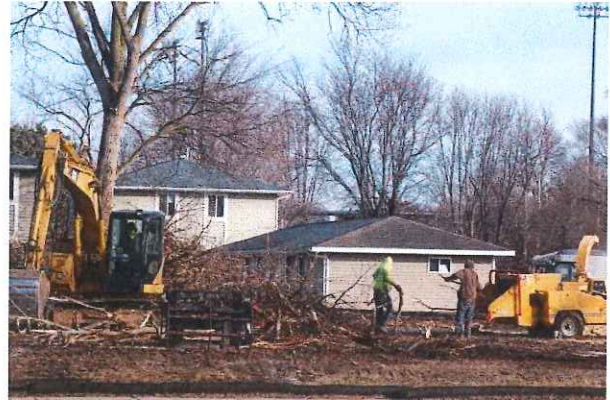
Austin Montgomery/Beloit Daily News Crews continue to clear the site near Telfer Park on Cranston Road. The site will be home to an assisted living facility.
